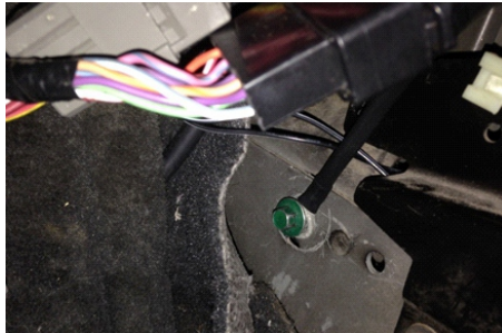
Figure 3 - Patch Loom Ground
